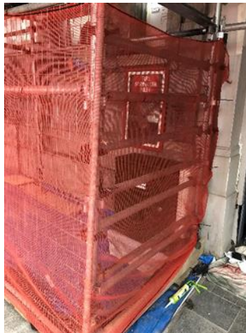
Figure 4 – Building refurbishment that hasn't considered panel/inlet access
