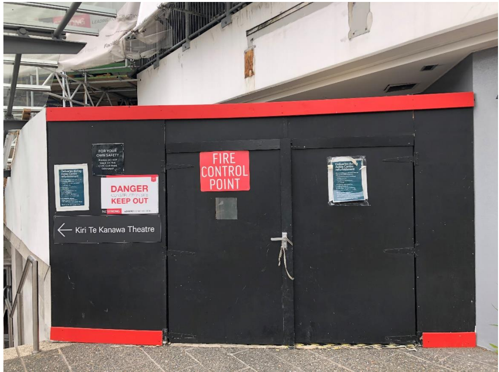
Figure 5 – Clear signage and access to fire systems on a refurbishment site
