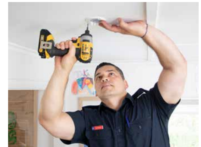
Our Home Fire Safety Team installs smoke alarms into eligible homes. We know working smoke alarms give people an early alert to fire in their homes, and the best chance of escaping alive.
