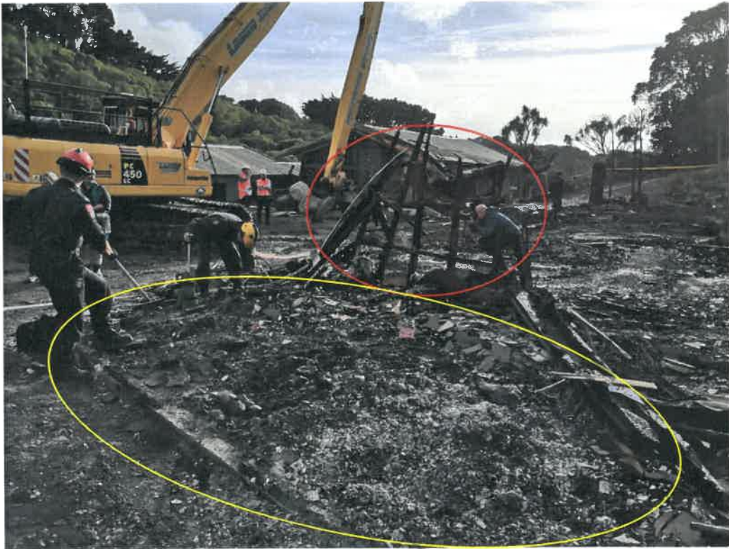
Photo 9 showing remaining wall (circled red) of adjacent bedroom. While the rest of the site had been cleared by an excavator, the area around the storeroom (circled yellow) had been preserved for further inspection.
