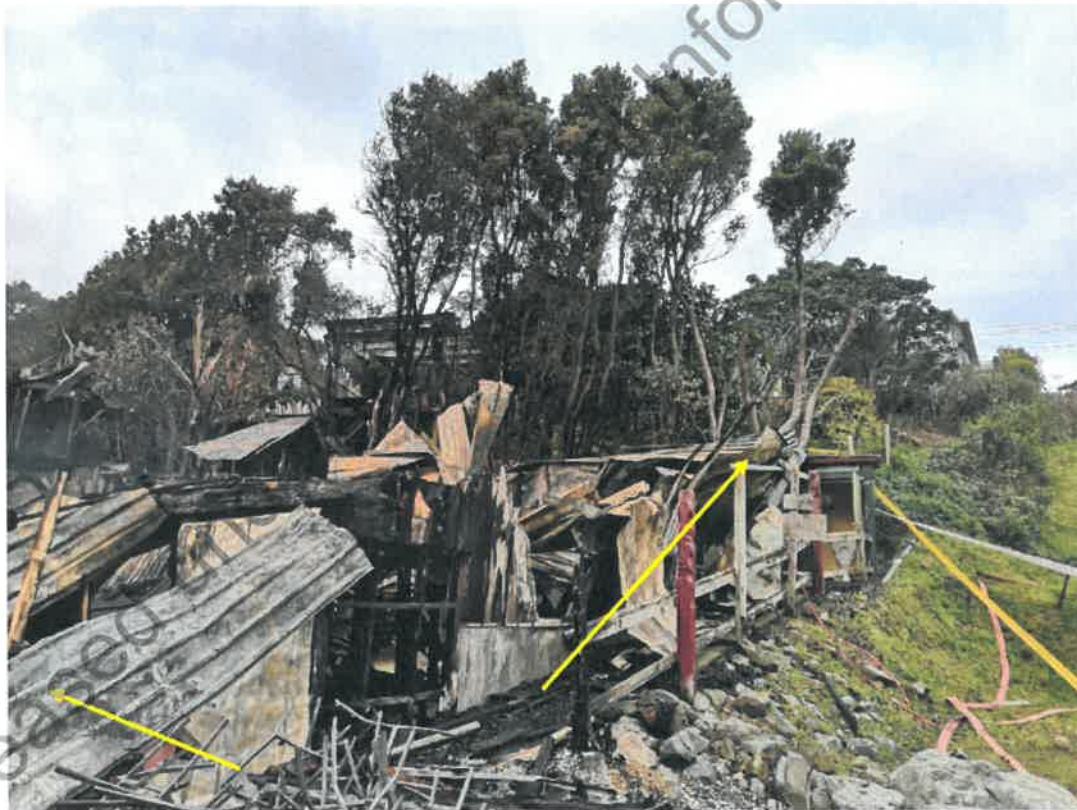
Photo 5. The arrow shows the directions of fire travel from southwest corner of building (location of a storeroom).
