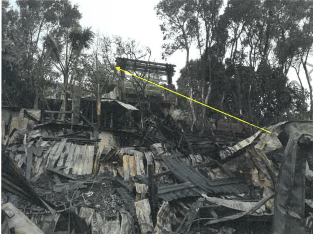
Photo 6 looking across the main house site from the west to the east side of the building, burn patterns show fire travel from the right to left of the photo (southern side of the building towards the north).
