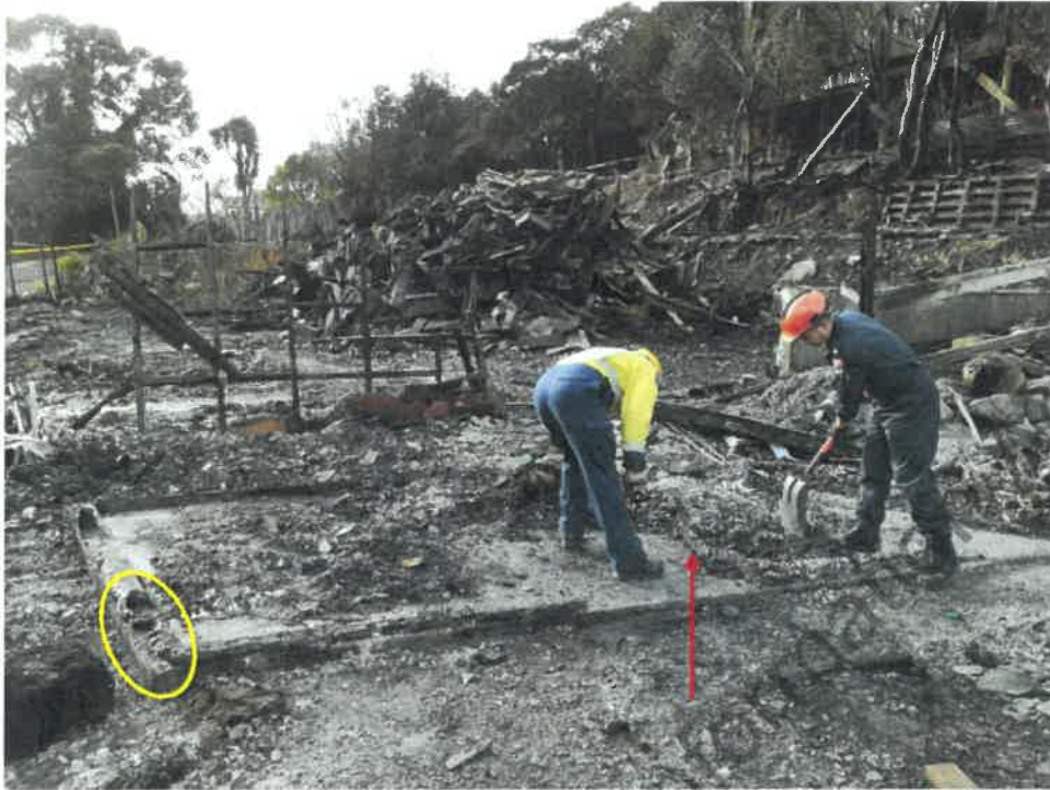
Photo 11 showing storeroom during continuing excavation. The red arrow indicates the remains of the door showing it was in the open position at the time of the fire. Witnesses stated the door was always left open.
