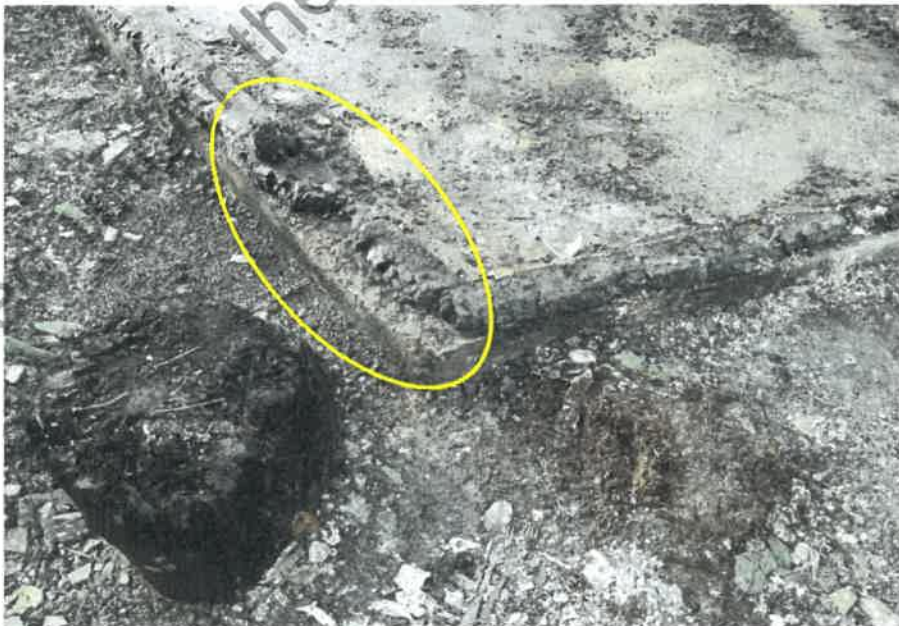
Photo 12 showing deep level charring of base plate on the south western corner of the storeroom.
