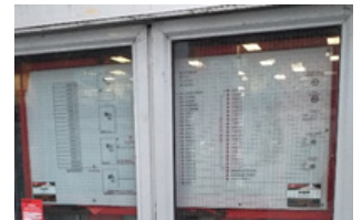
Fire alarm panel.
