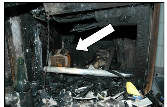
Right: The "Smoking Gun" The remains of the roller door is visible still resting on the toaster switch.
