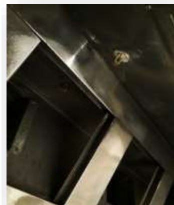
Figure 3- Sprinkler above fryer
