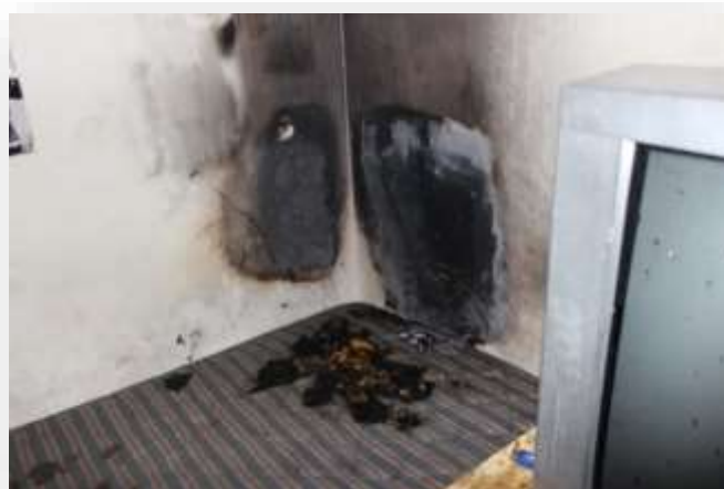
Photo above shows hostel apartment with small fire suppressed by a sprinkler activation.
