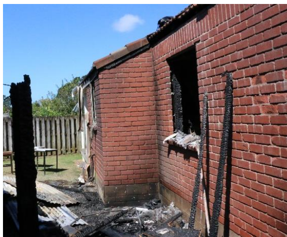
Figure 2 – Fire damage to house on same property
