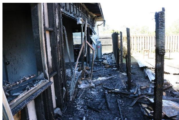
Figure 1 – Fire damage to fence and neighbouring property
