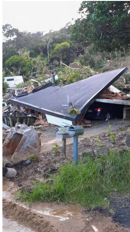
Figure 8 above. CFO rescued a person from underneath the roof section shown above. This is the roof of the centre-front house shown in figure 7 above. (USAR Photo)
