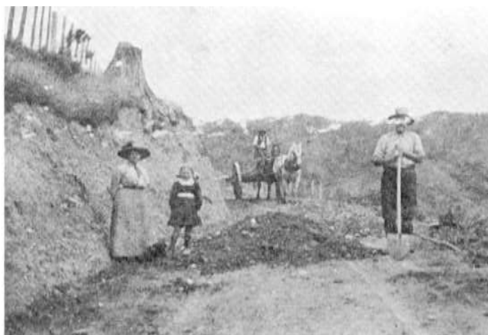
Work on the Wainuiomata Hill Road c 1911. Again the lack of vegetation is clear but stump shows it was recently forest
