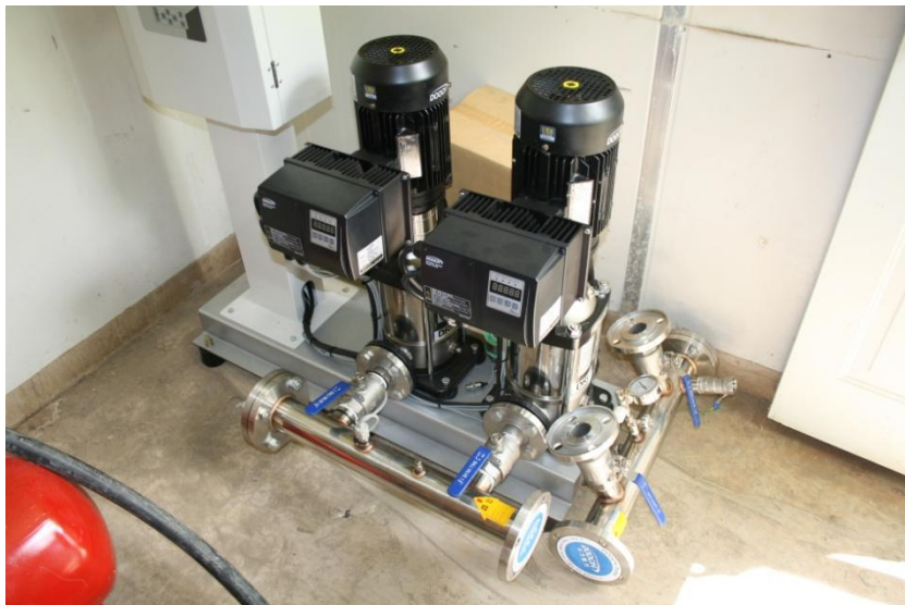
Figure 16: Double electric pump system
