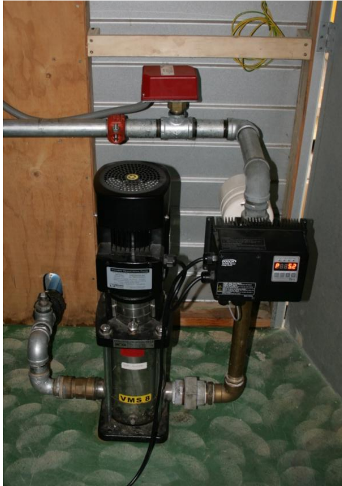
Figure 15: Single electric pump
