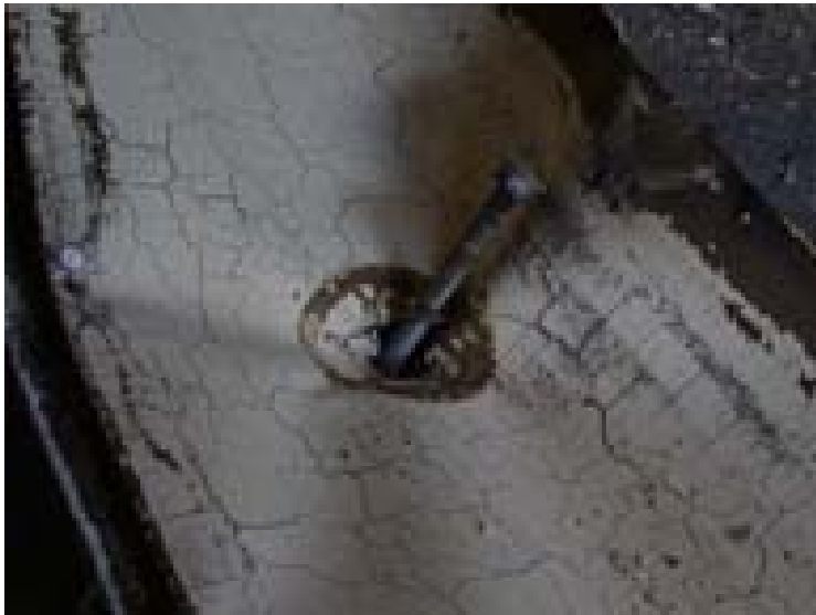
Figure 4.59: Cupping around hanger point.
