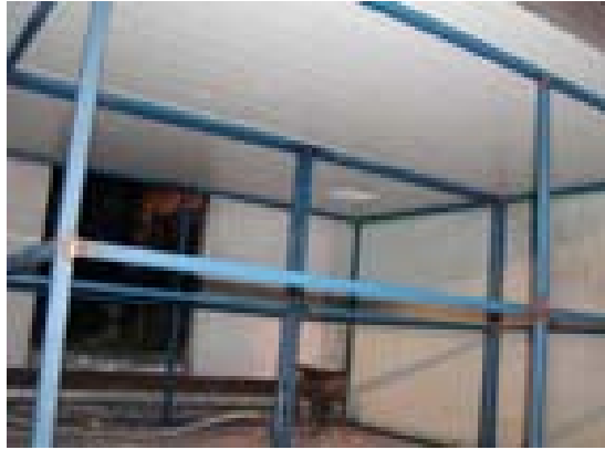
Figure 4.17: Location of burner and cut out in panel.
