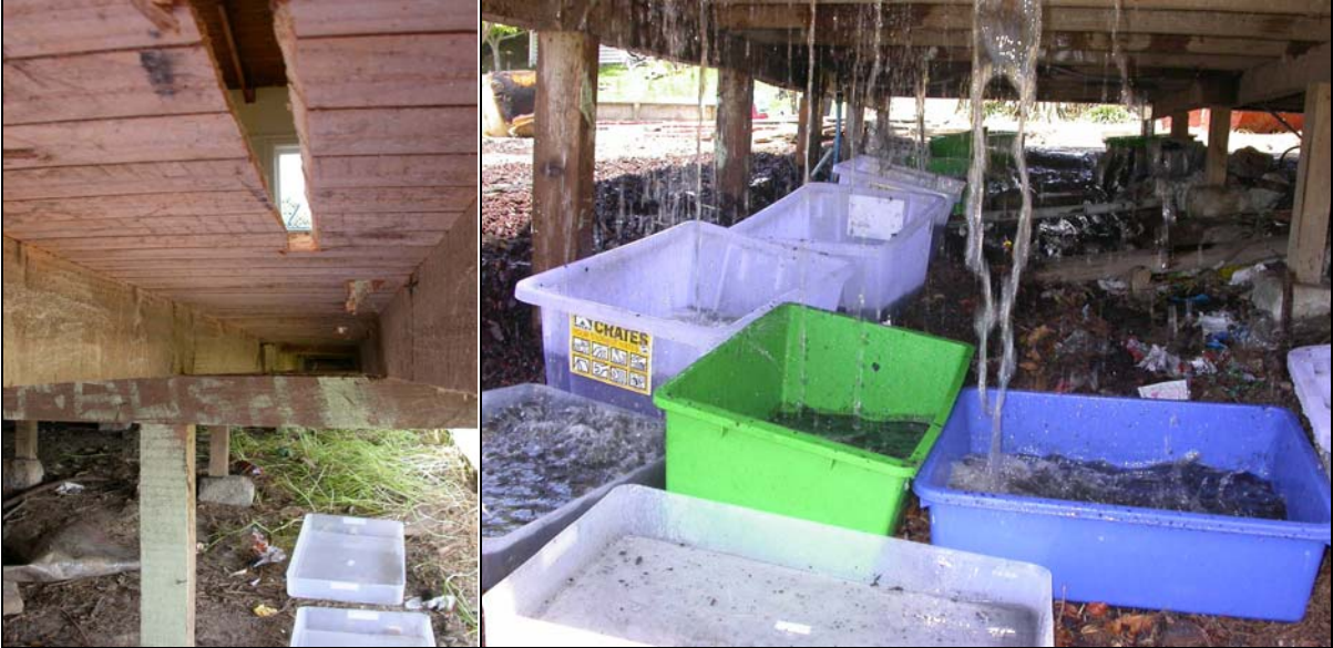
Figure 3: Fire-water collection below the St Mary's School tennis shed. Left: Holes cut into the floor allowed collection of fire-water beneath the shed. Right: Fire-water draining into plastic bins placed below the drainage holes.
