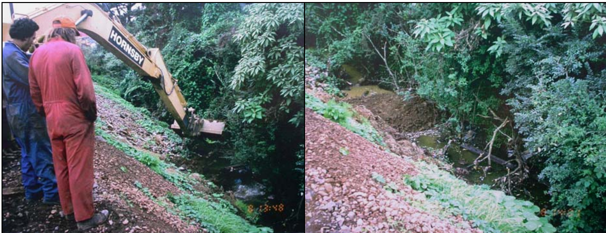
Figure 22: Otahuhu Chromeplaters Ltd, 7 – 8 May 2000. Left: Construction of an earth dam in the stream to intercept contaminated fire-water. Right: Completed earth dam retaining fire-water, allowing removal of contaminated water by Chemwaste sucker trucks. (Photos: Auckland Regional Council).
