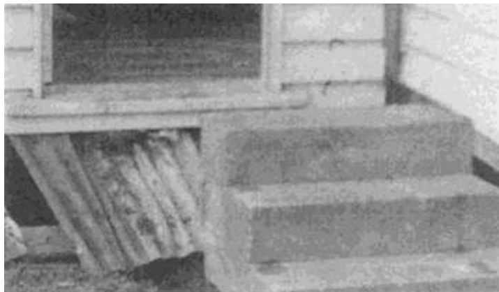
Figure 0-4 Full Piled Foundation slipped off Foundations, with Concrete steps remaining in place (Source: Cooney 1979)
