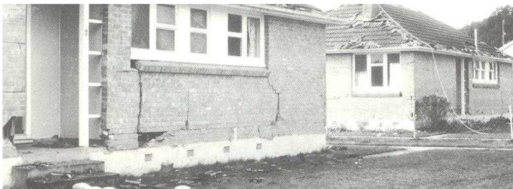
Figure 0-6 Superficial Damage to brick veneer on State Dwellings, however no damage to the Foundation Wall is evident (Source: Eiby 1980)
