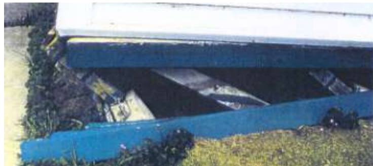
Figure 0-2 Corner of Foundation showing Piles swayed to one side (Source: BRANZ 2003)
