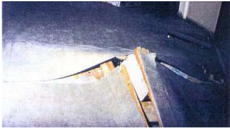
Figure 0-3 Example of Piles punching through the Floor due to Sub-floor Framing slipping off Piles (Source: BRANZ 2003)
