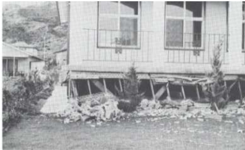
Figure 0-7 Jackstudded Sub-floor showing Cladding broken off and a slumping to one side (Source: Jennings and Housner 1971)
