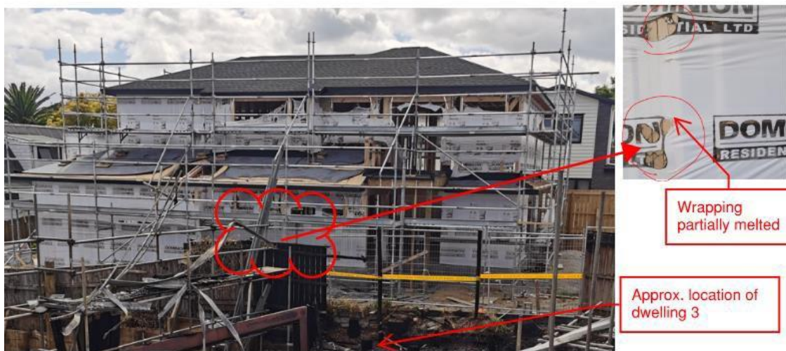
Figure 11: Extent of damage neighbouring properties under construction from the east
