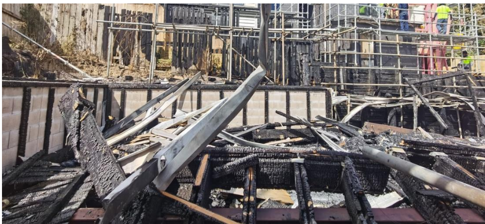
Figure 7: The extent of damage to Dwelling 3 – View from North (entry access way)
