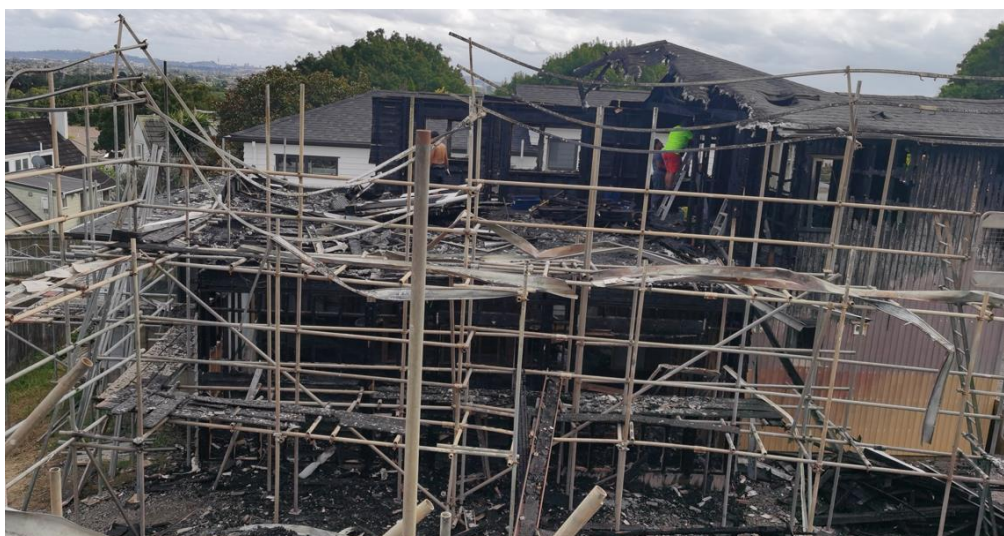
Figure 8: The extent of damage to Dwelling 2 – Overlook from South
