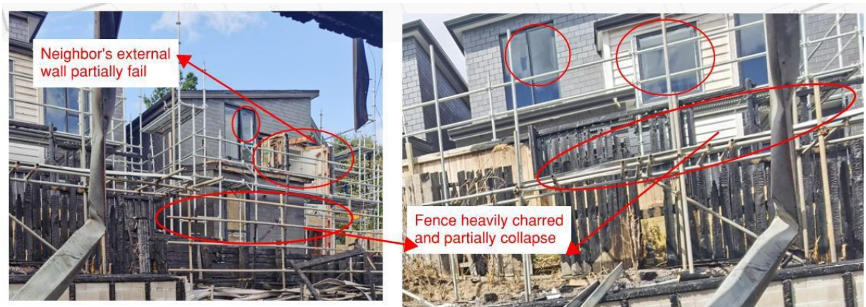
Figure 10: Extent of damage neighbouring Redoubt Rd subdivisions at the rear
